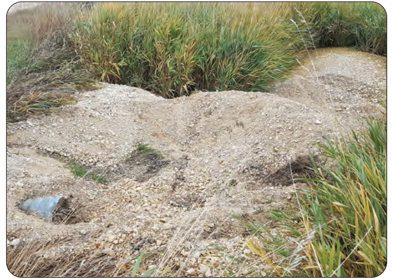
Culverts and drains remain plugged.
