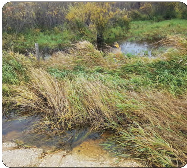
Overland flooding water still remains trapped on farmland because of plugged drains and culverts.
