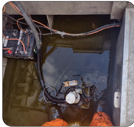
Algae choking the pump had to be cleared out.
