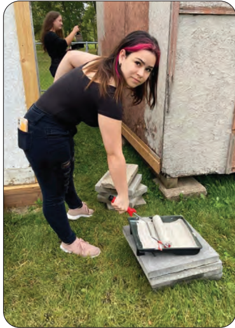
A volunteer helps paint a shed, which the Bayview Church in Gimli offered to house on its site.
