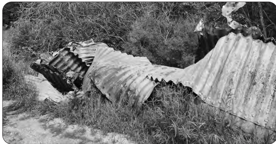
The damaged culvert was dug out of the Drunken River and left on the side of the road, posing a danger to children. As of last week, it was still there.
