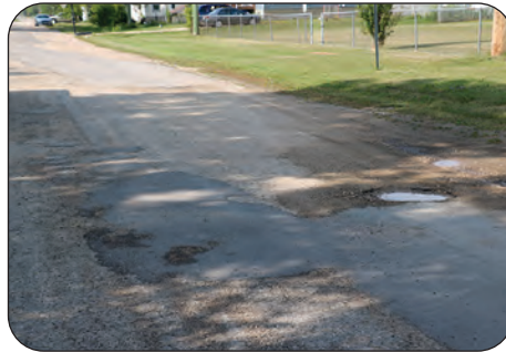
Fifth Avenue, like Sixth, has patches of asphalt, potholes and gravel.
