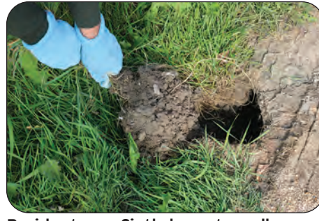
Residents on Sixth have to pull grass, weeds and clumps of mud from a collapsed culvert to prevent possible flooding of their property.
