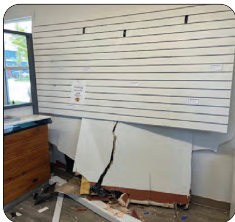
The inside of the club shows the breached wall in the public gallery section of the building.
