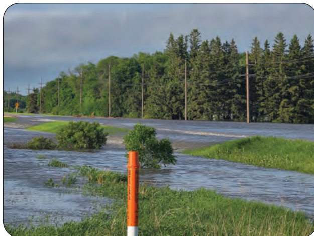
Highway 9 at Matlock as well as Pike Road is washed out.
