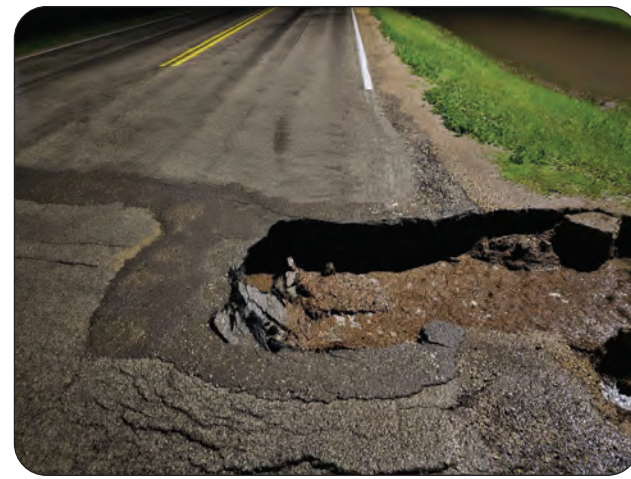
Southbound on Gimli Road in Matlock at Bubbling Well Rd. This hole is 2 feet deep.
