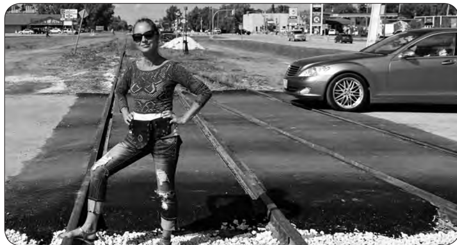
The crossing at Gimli's Rona store had vehicles practically sailing over the tracks. A driver checked out the repairs.
