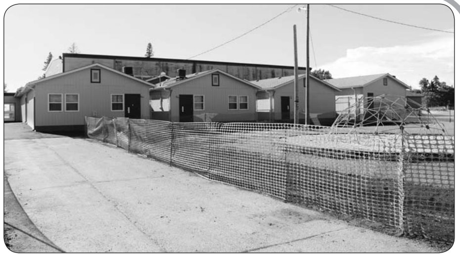
Three of the four huts at Dr. George sustained water damage in 2015
