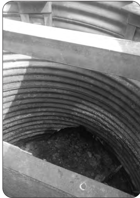
A concrete block inside the control structure was lifted by someone a few years ago, draining the wetland "almost down to nothing."
