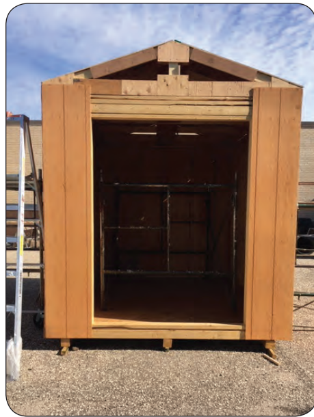
Lundar High School Grade 10 Industrial Arts students are building a shed for the Lundar skatepark.
