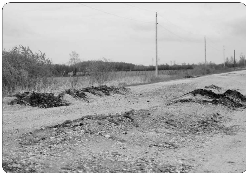
Along Road 97N, just east of Highway 6 between Laurentia and Johnson beaches, a number of frost boils have breached the road.
